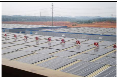
World's Largest Roof Top Solar PVS System
